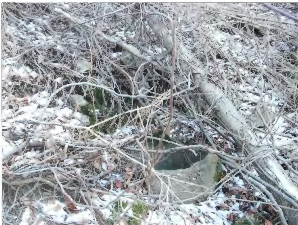
Figure 5.86. Concrete pipe on north slope of Battery Kingman. The concrete pipe should be capped to prevent possible injury and reduce water entering into or around the underground structures (Olmsted Center, January 2009).
